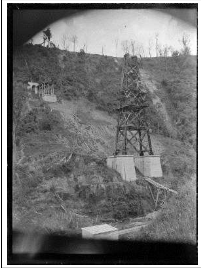
Figure 1: View of the Makohine Viaduct under construction, ca 1900. Godber, Albert Percy, 1875-1949: Collection of albums, prints and negatives, ATL, APG-0021-1/2-G
