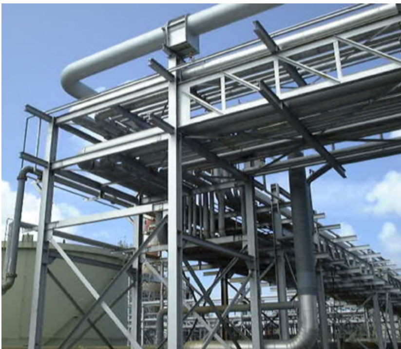
Figure 4: Pipe rack and pipe bridge.
