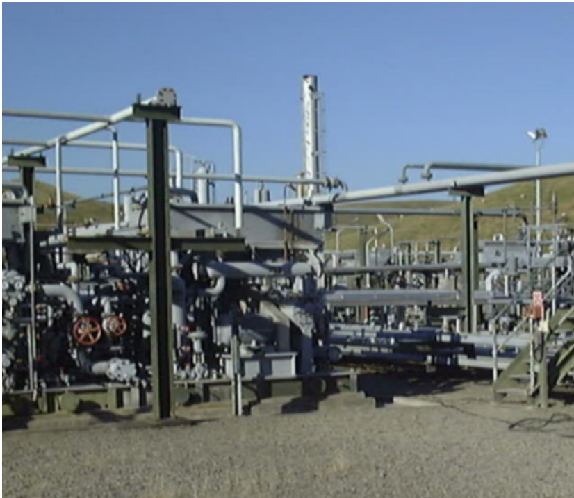
Figure 12: Pipes and pipe supports.
