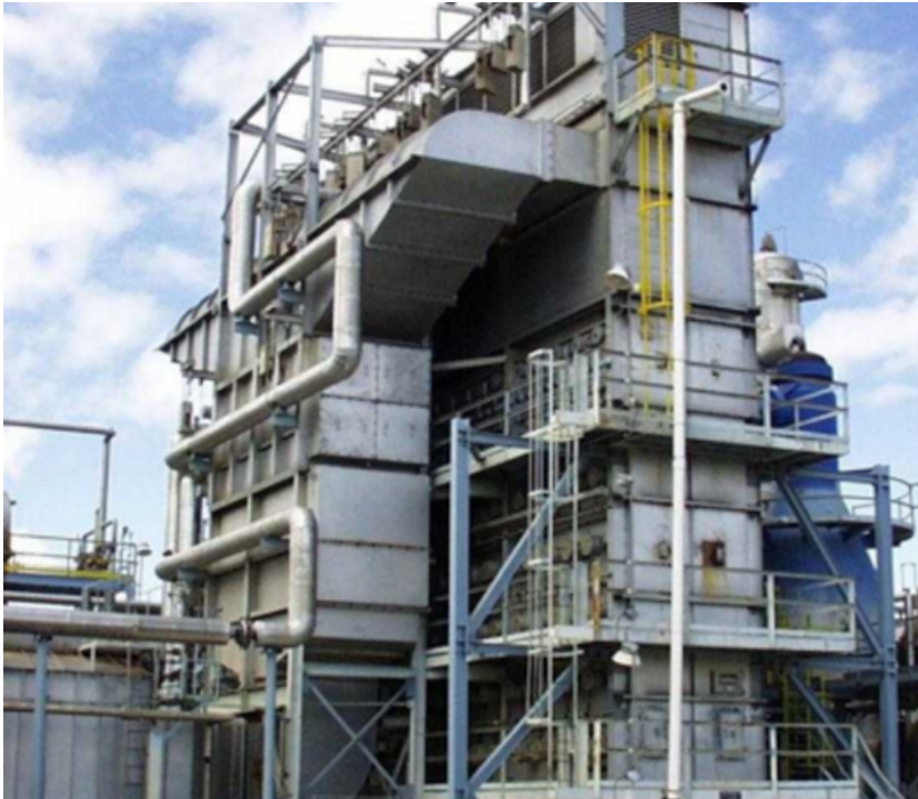
Figure 9: Vertical fired heater.
