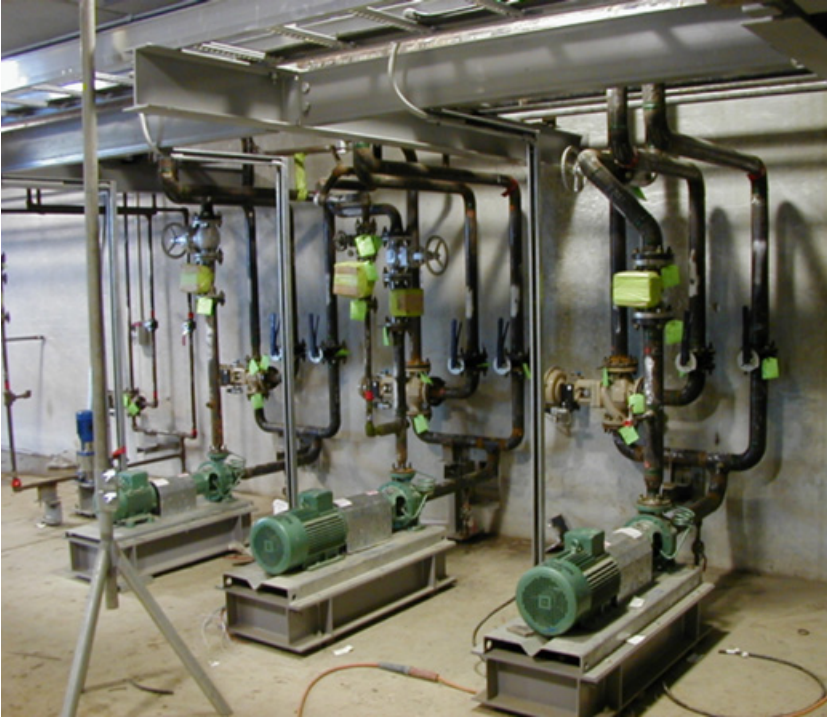
Figure 5: Rigid structures – pumps skid mounted at grade.
