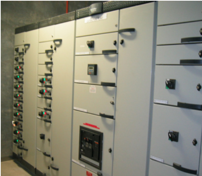
Figure 10: Floor mounted cabinets.
