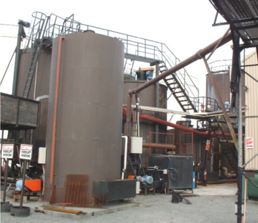
Figure 6: Flat bottomed tanks.
