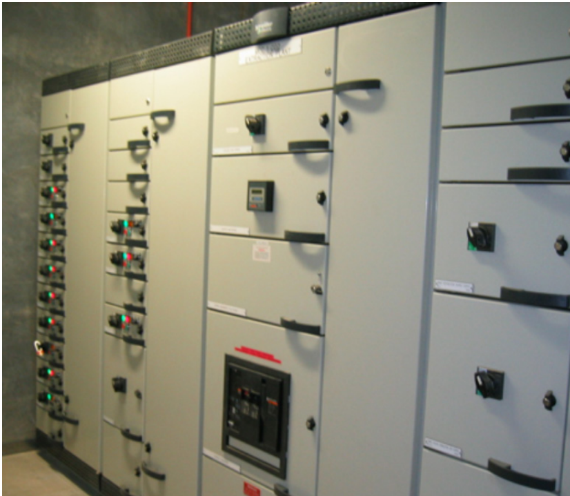
Figure 10: Floor mounted cabinets.
