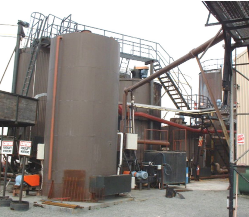
Figure 6: Flat bottomed tanks.
