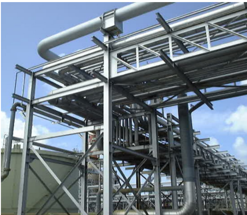
Figure 4: Pipe rack and pipe bridge.
