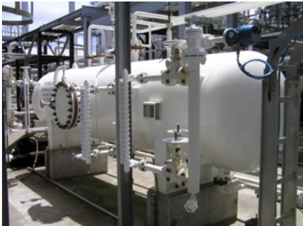
Figure 1. Horizontal pressure vessel on short pedestals
