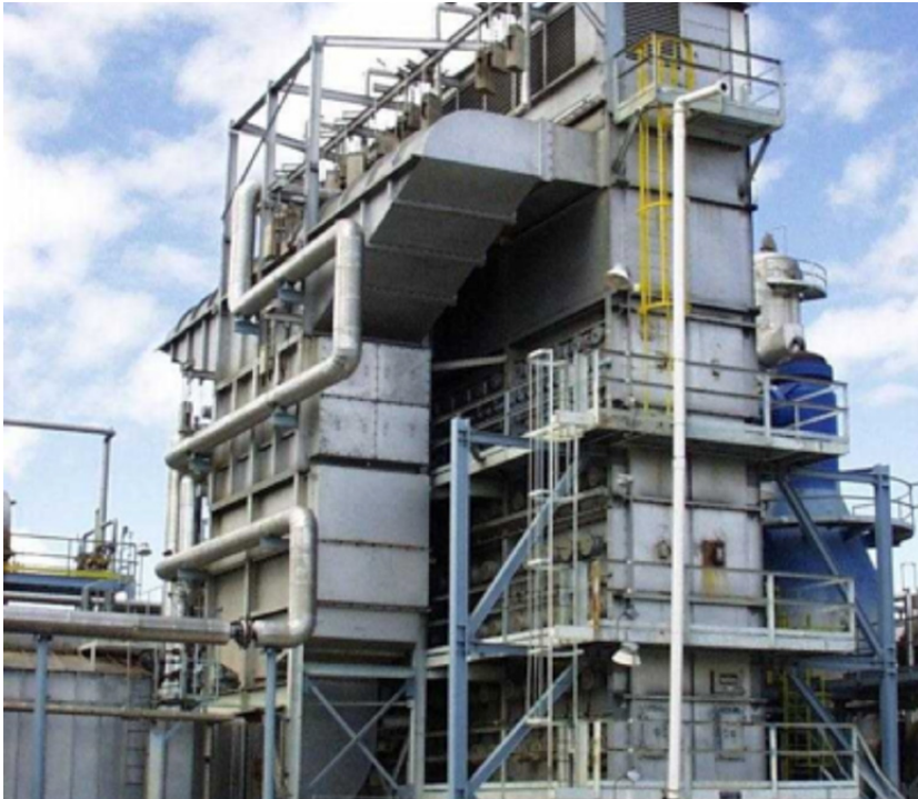
Figure 9: Vertical fired heater.
