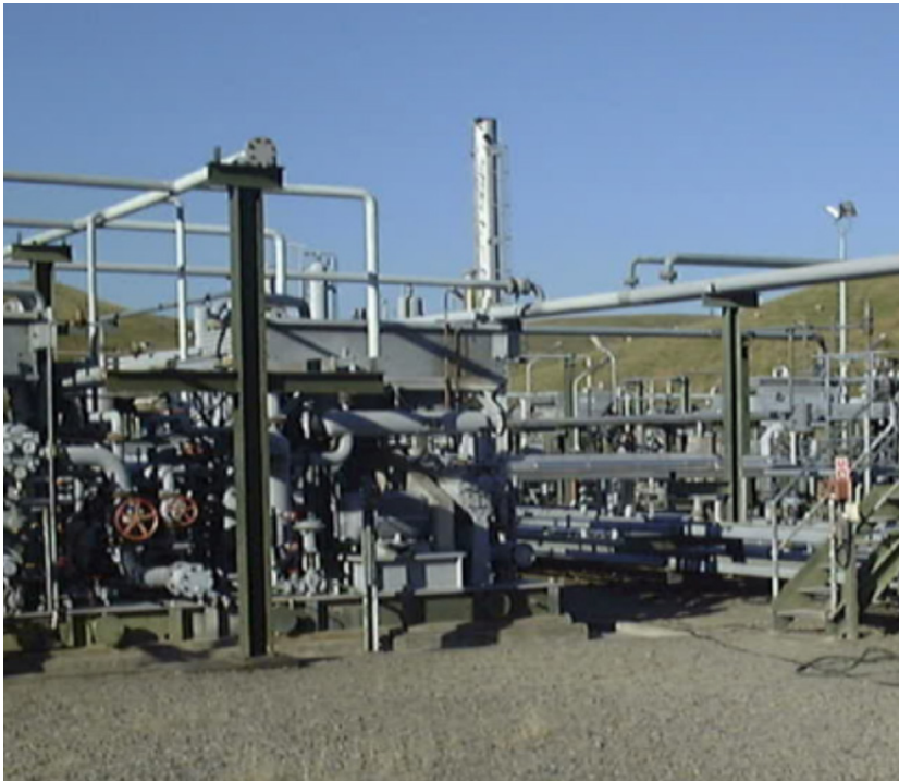
Figure 12: Pipes and pipe supports.
