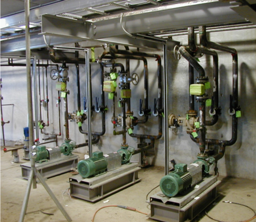
Figure 5: Rigid structures – pumps skid mounted at grade.
