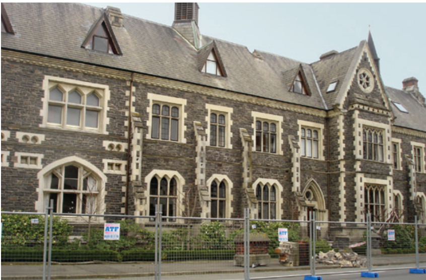
The damaged Old Normal School, photographed on 16 September 2010. Photo: Kete Christchurch.
